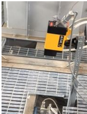
↳ Strip loop control in furnace
